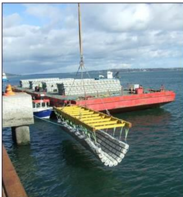
Figure 7-14 An example of concrete mattresses to be used to stabilise dredge slopes in the Berth 53 area
